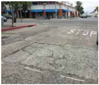
Failing broken and degraded concrete panel.
