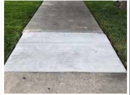
Finished repair with a new lifetime of service. Open for use within two hours of placement.
