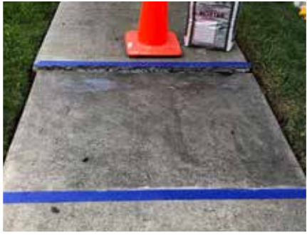
A trip and fall liability hazard.
