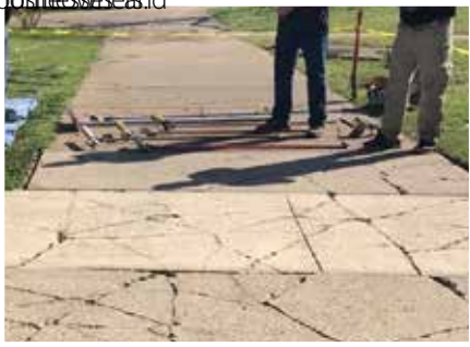
A severely cracked and degraded sidewalk.
