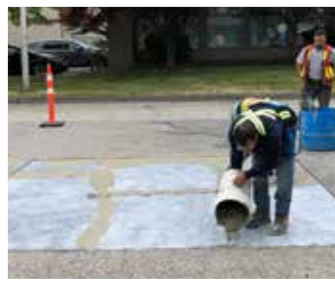
The area is primed with Yeti Armor™ Primer and large cracks filled with Yeti Armor®.
