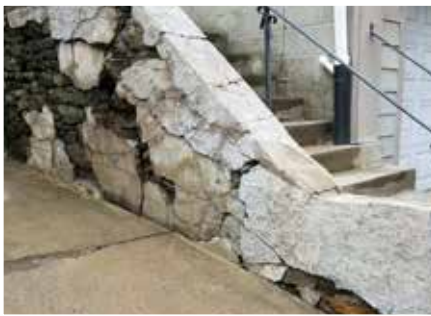
Severely degraded vertical wall.
