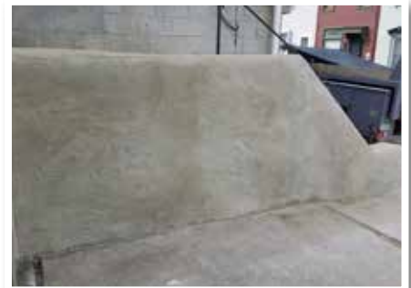
The degraded wall has been given a new life cycle and a brand new appearance.
