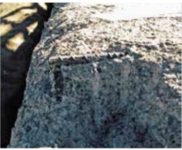
Spalled concrete with exposed rebar.
