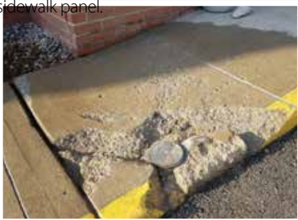
Severely degraded sidewalk causing trip hazard.
