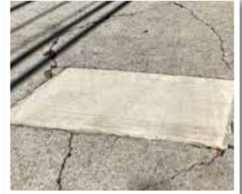
Spall repair one year after placement.
