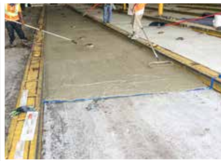
Yeti Armor™ overlay is rolled and finished over existing primed concrete to a thickness of 1 2".
