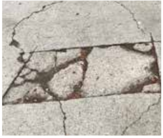
Cracked and spalled concrete.
