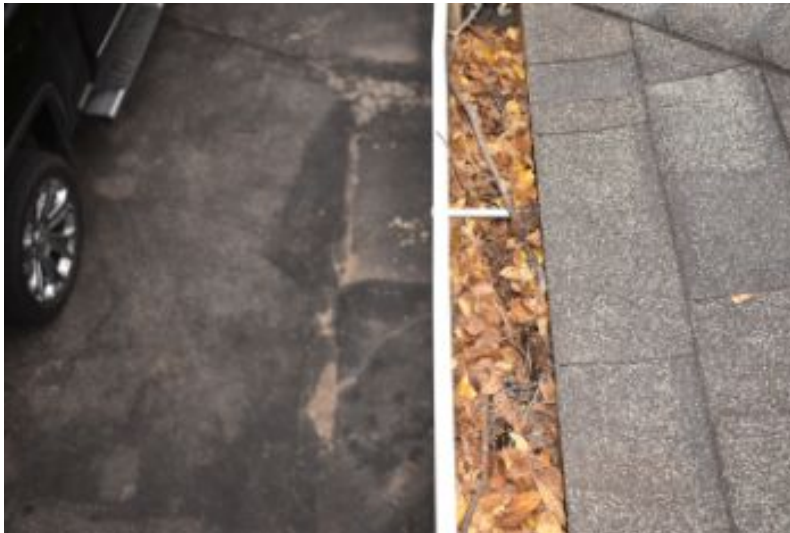
Clean gutters: Significant amounts of debris evident.
