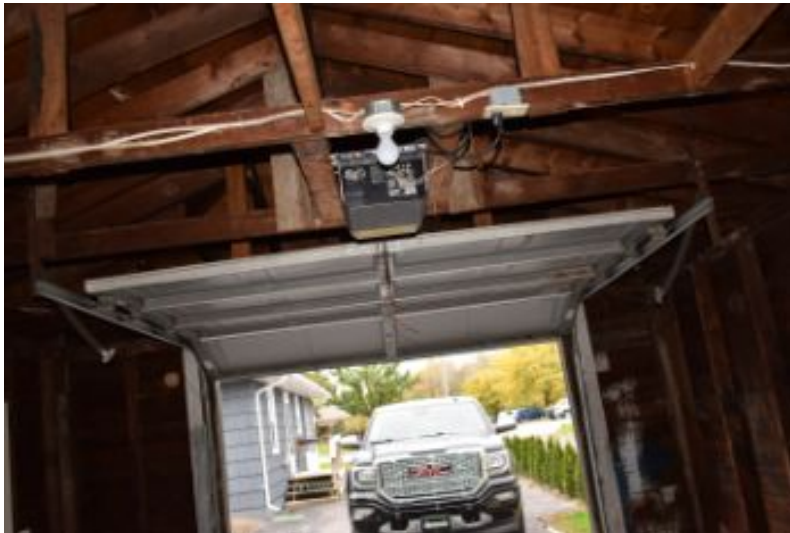
Chain drive opener noted.
