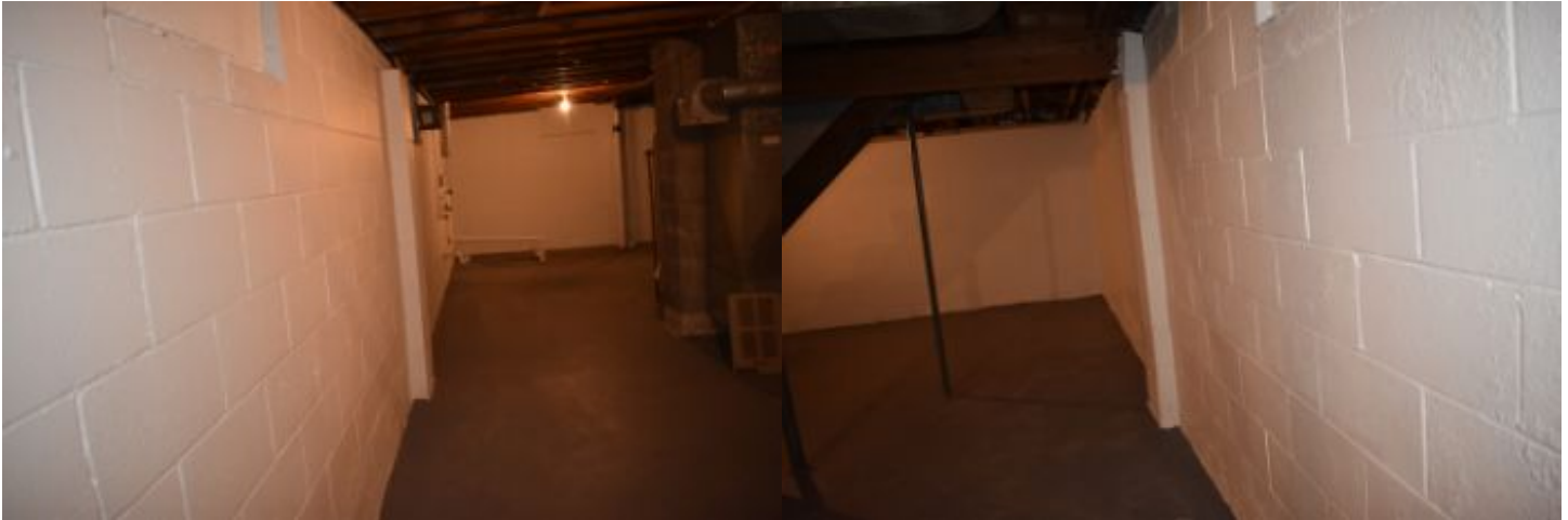
Readily Visible portions of foundation wall appeared serviceable and dry at the time of the inspection. See Limitations.
