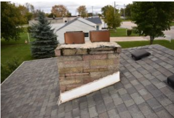
No chimney cap visible from inspection level. Recommend installation to prevent premature weathering and water intrusion
