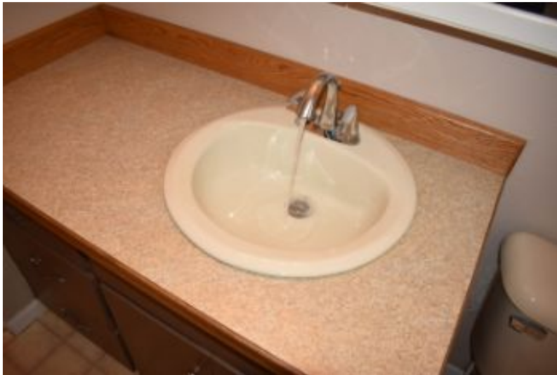
Sinks operated normally at time of inspection.
