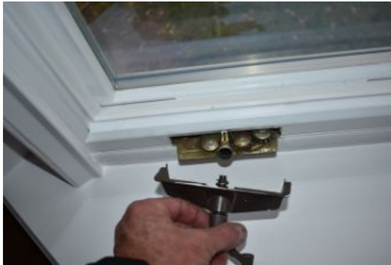
Broken crank noted at front south window.
