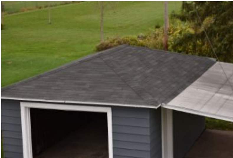
No major system safety or function concerns noted at time of inspection.
