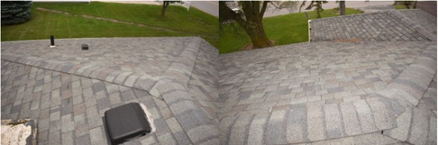
Older shingles noted in fair condition. Estimated remaining serviceable life: Over 5 years.
