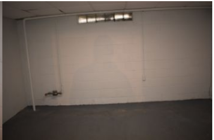
Readily Visible portions of foundation wall appeared serviceable and dry at the time of the inspection. See Limitations.
