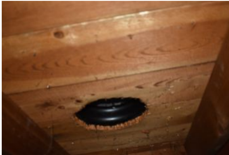
Fixed, roof-field exhaust vent noted.
