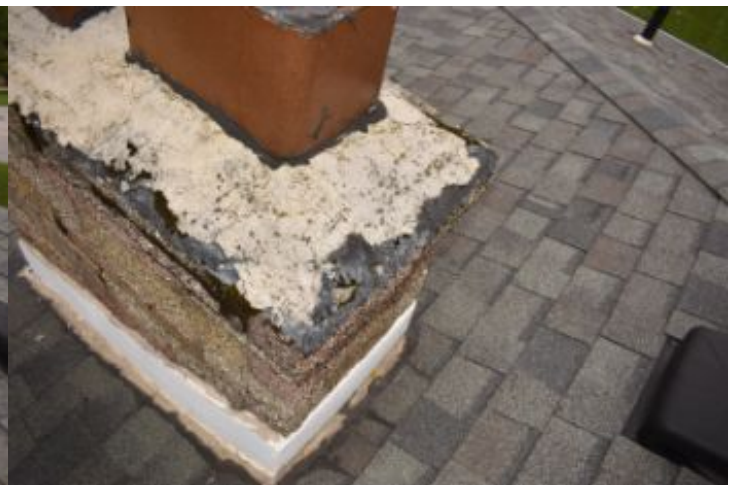
Chimney crown should be re-sealed.
