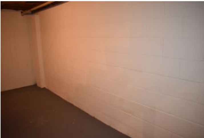
Readily Visible portions of foundation wall appeared serviceable and dry at the time of the inspection. See Limitations.
