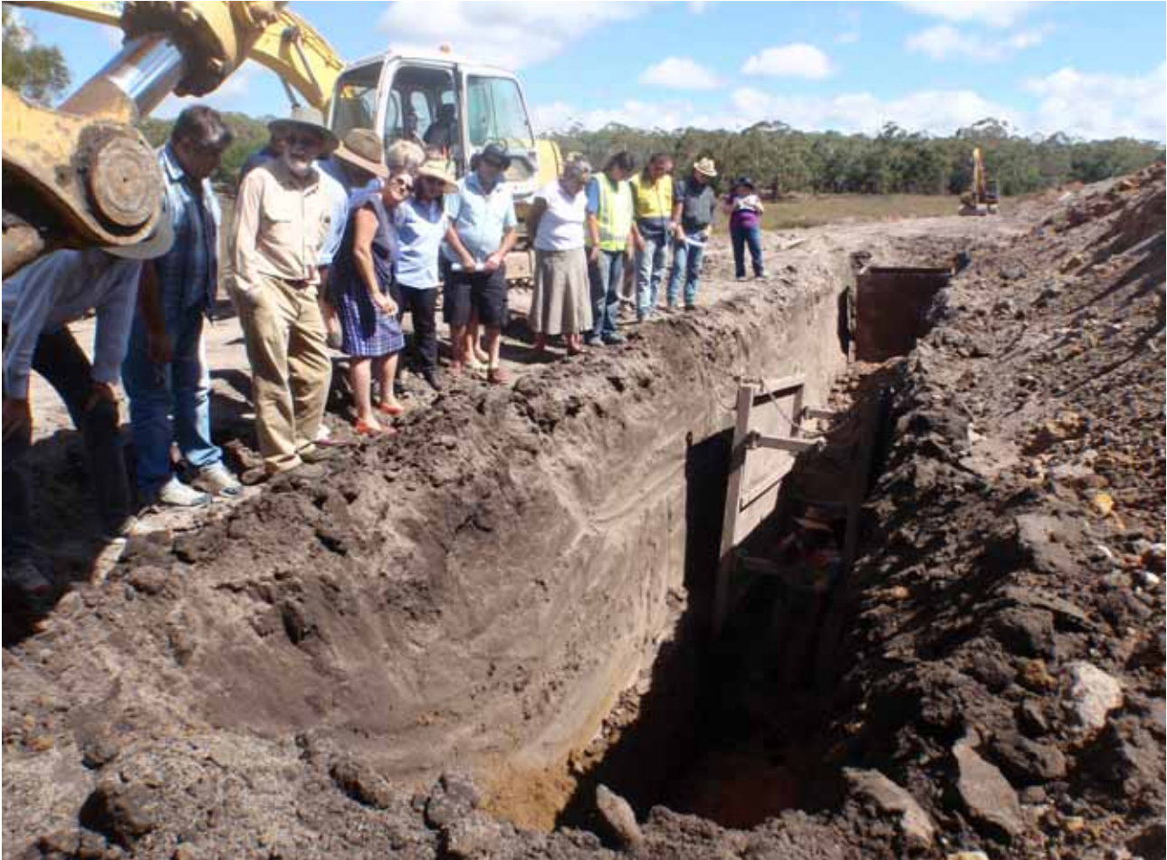
2.82 Lake Condah Sustainable Development Project members viewing the construction of the regulator gate on the cultural weir at the downstream end of Tae Rak, March 2010
