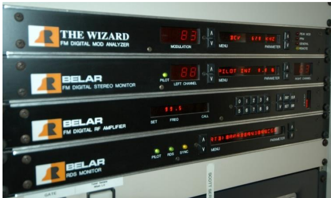
Fig 2 Array of modern FM modulation monitors that have remote control capabilities
