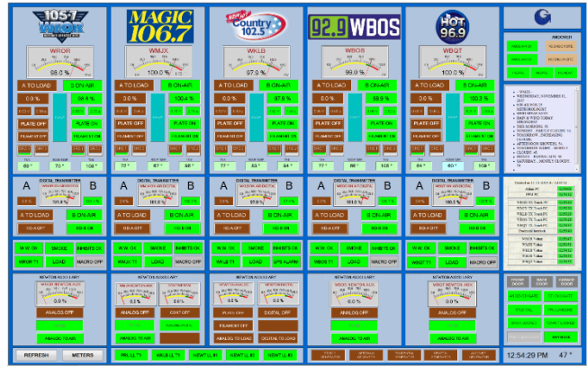
Fig 7 This screen allows for control as well as monitoring on one screen. Using a cursor, the buttons can control relays at the remote site.
