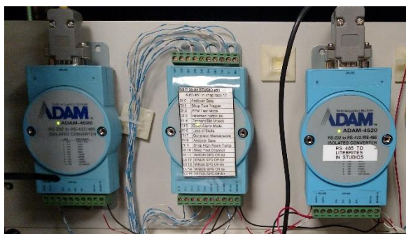
Fig 3 In this case data acquisition modules are mounted to a rack panel and wired to status and analog inputs. These modules are addressable on an RS-485 data bus
