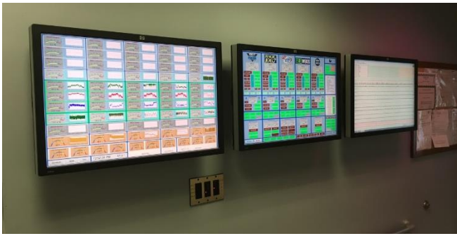
Fig 5 One entire wall dedicated to displaying status and analog values
