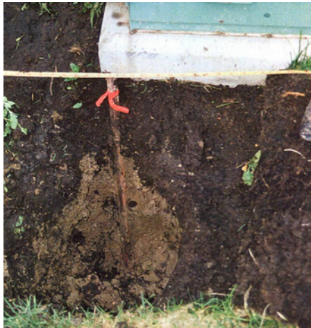
Fig. 1 – Boundary monument beneath utility box and concrete slab
