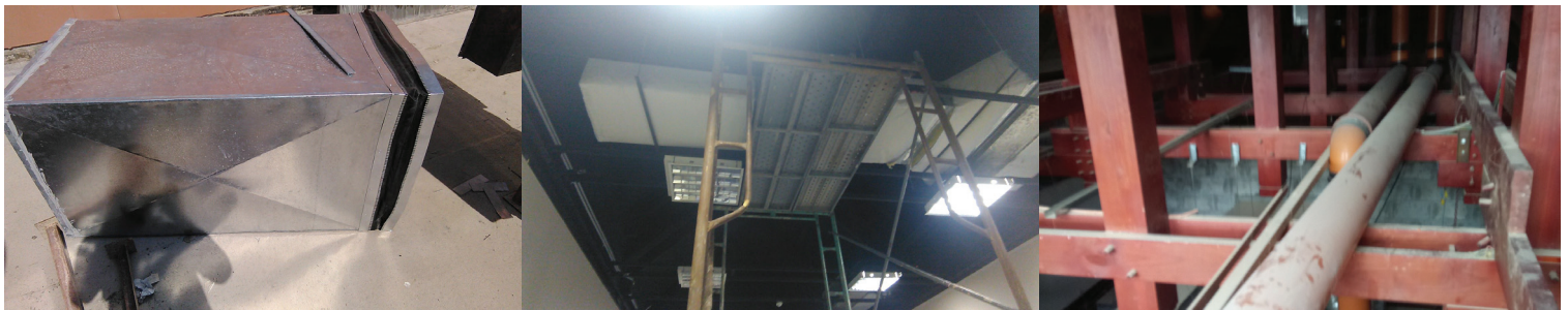
Bushido Restaurant – MEP Works
