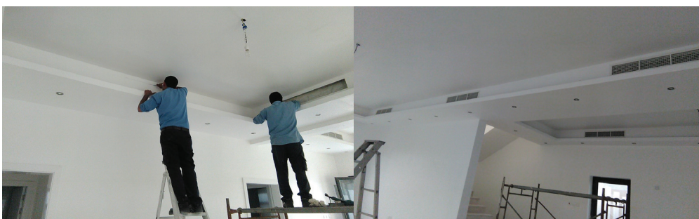
Private Villa @ Askar – MEP Works
