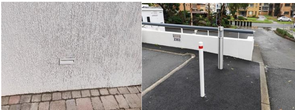
Figure: Inset wall lights and bollard lights.
