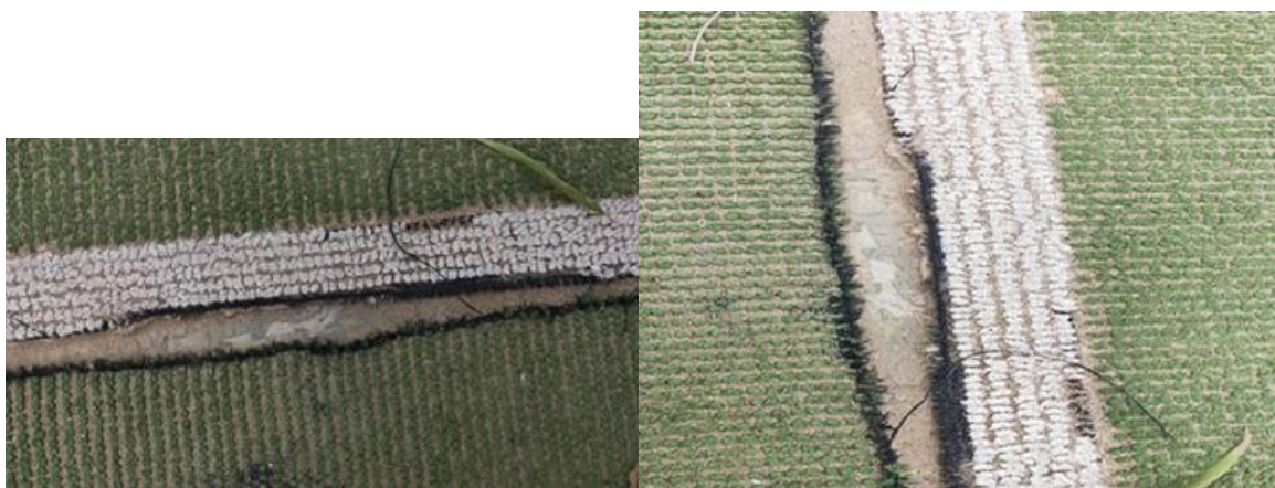
Figure: Some of the tears in the tennis court surface
