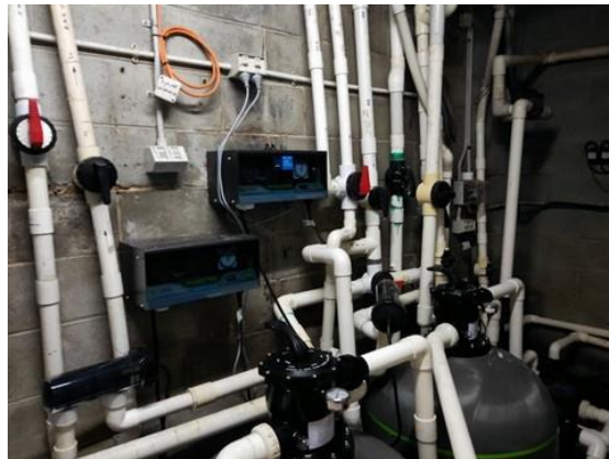
Figure: Pipework in pool room before reconfiguration.
