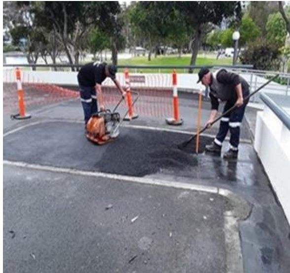
Figure: Pavers removed to stop water ingress.
