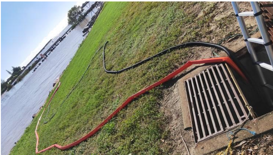
Fire sprinkler Reserve Storage tank
