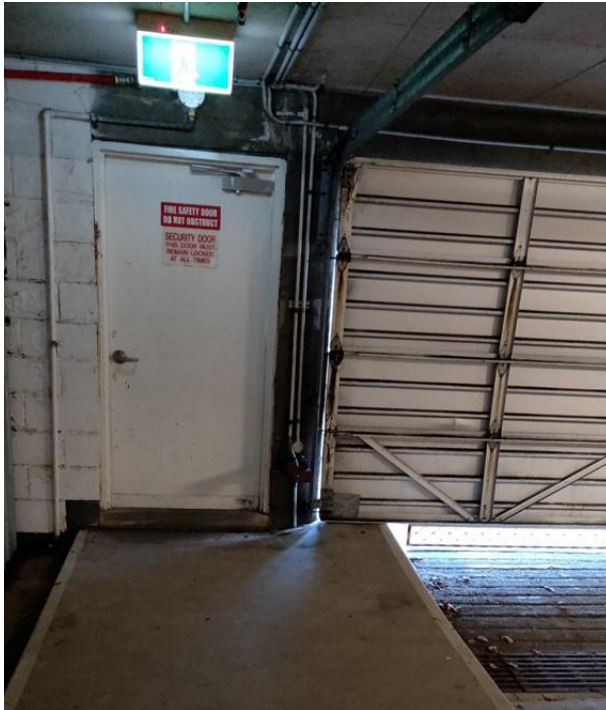
Figure: The concrete slopes away from the drain allowing water to enter the basement
