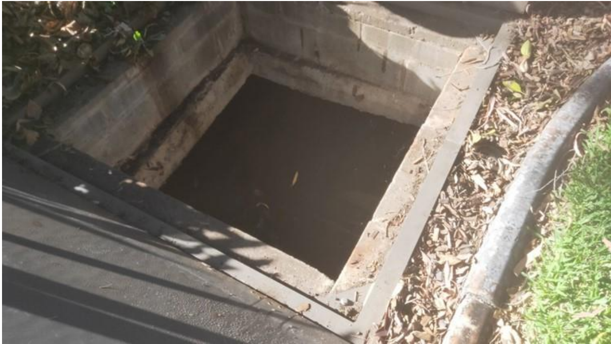
Figure: Water well above the float valve which cannot be seen in the picture
