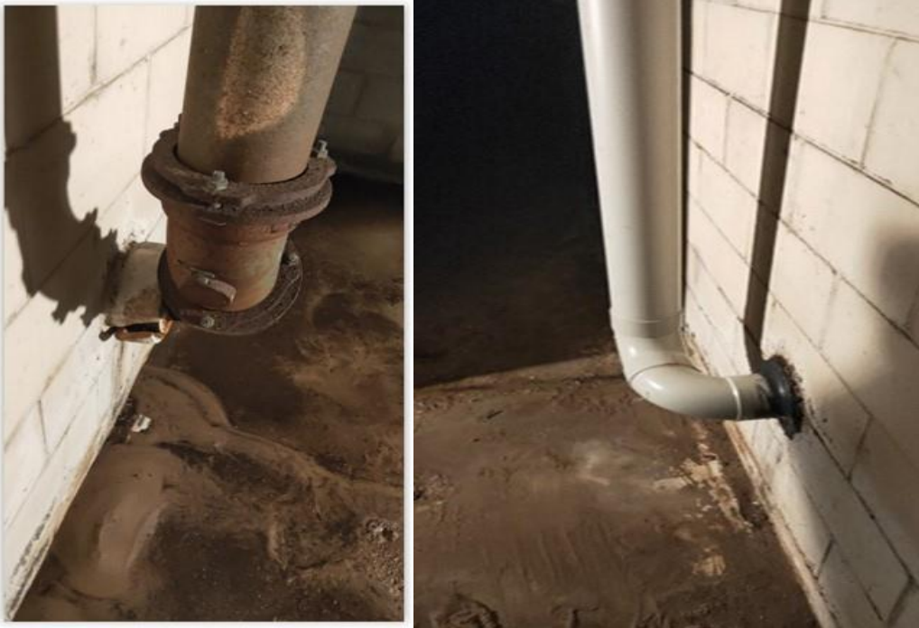
Figure: The offending pipe and the completed repairs.
