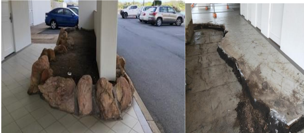
Figure: Old tiles with raised garden with no drainage
