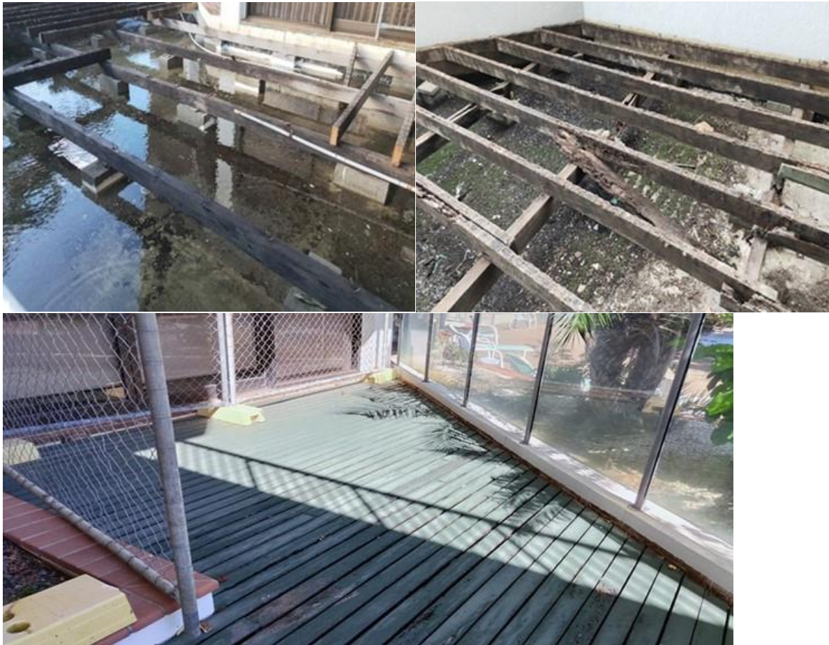
Figure: Old deck showing lack of drainage, rotten timber
