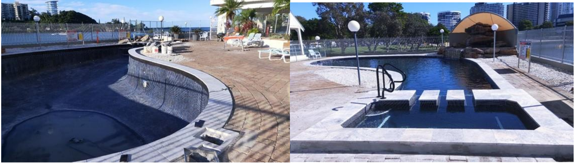
Figure: Pool leaking pipes and coping upgrade.
