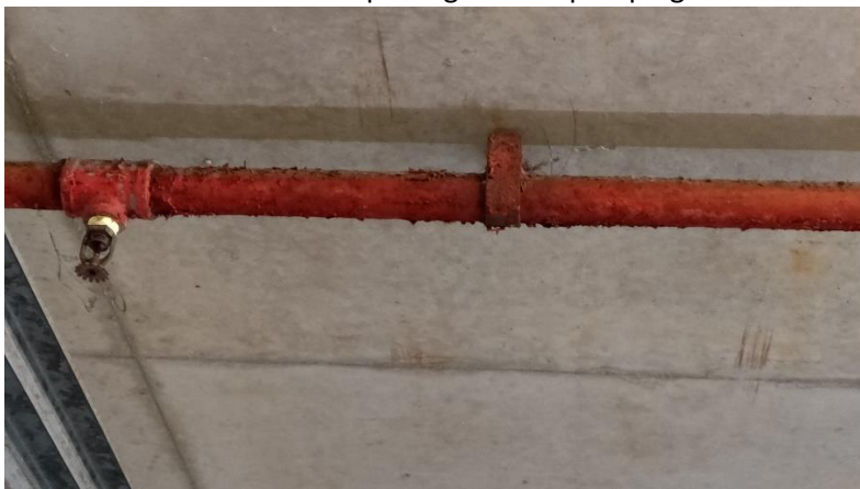
Figure: Rusted fire sprinkler pipe that needs to be replaced
