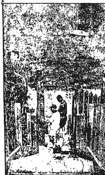
PATH TO THE WATER: Greg R... left, and Bill Snyder build a set of stairs to the beach near their homes.
