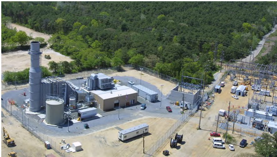
Brentwood Peaker Plant, 47MW
