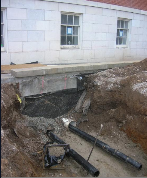
Supply and Return Lines
