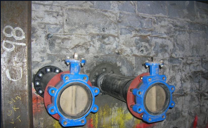
Supply and Return Line Penetrations Sealed and Fitted with Butterfly Valves
