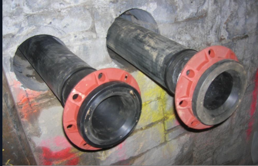
Interior Penetrations for Supply and Return Lines from Manifold Vault
