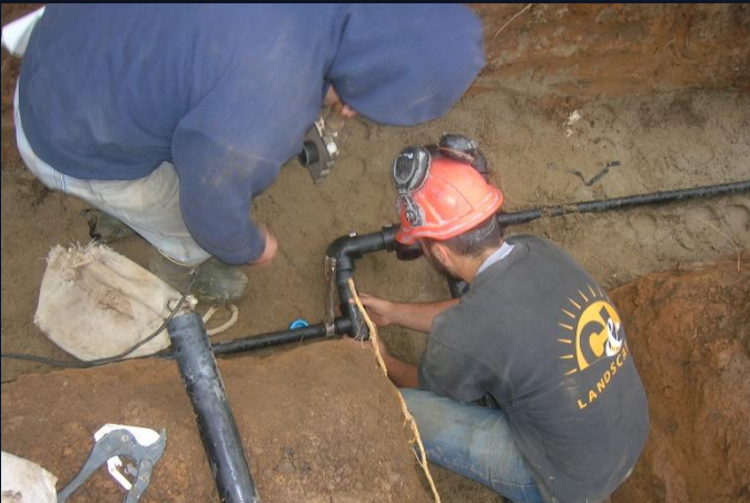
Horizontal Piping Assembly
