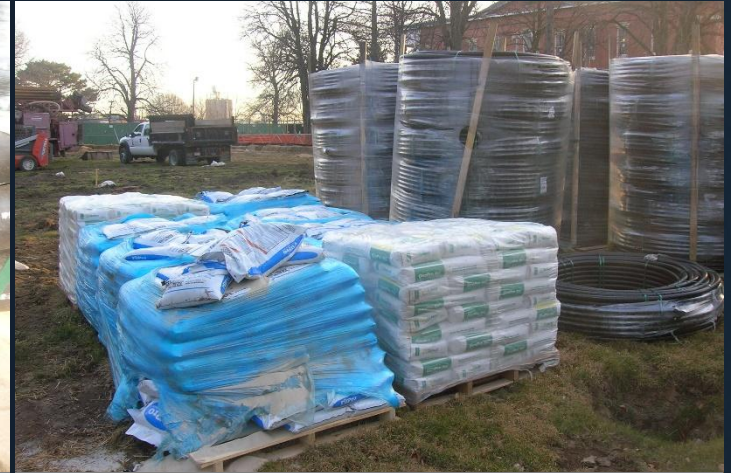
Grout Materials and Piping
