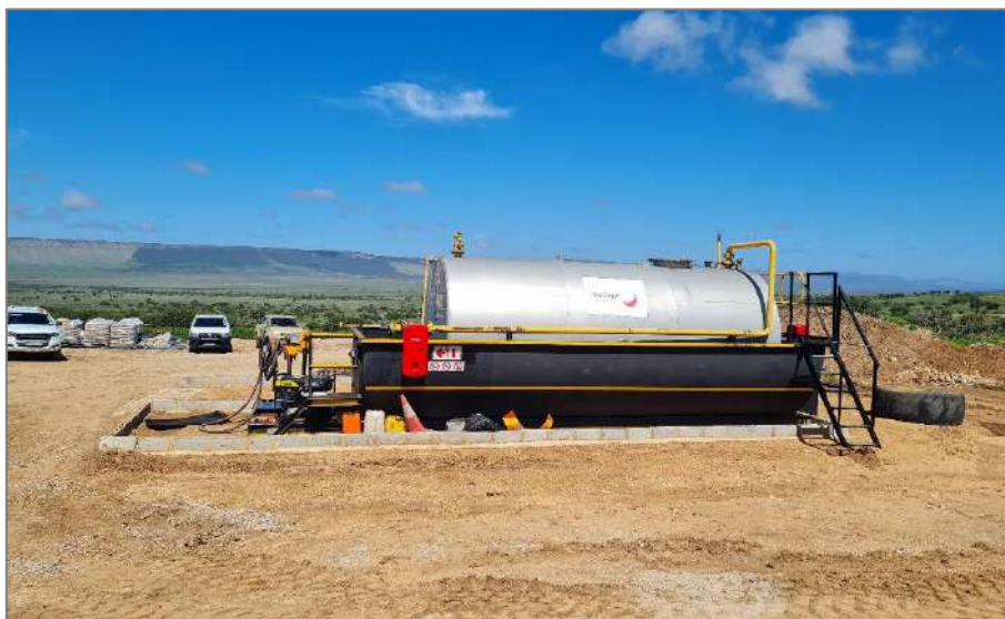
Figure 2: Bunded Bulk fuel storage area
