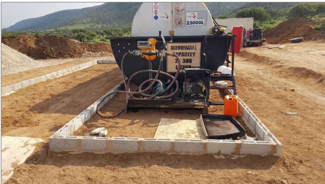
Figure 4: Self banded fuel storage with additional measure.
