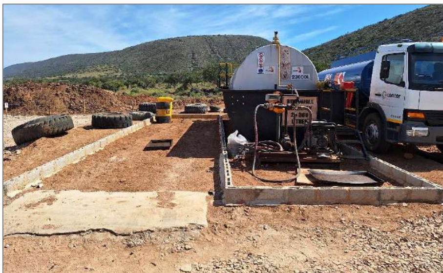
Figure 1: Self bunded bulk fuel with additional bunding measures in place.
