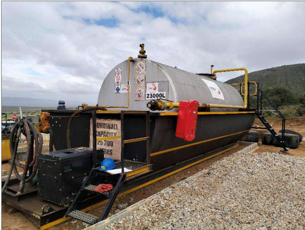
Figure 4: Bulk fuel storage with additional bunding.
