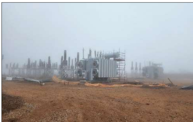
Photo 5a: Second transformer installed at the substation.
