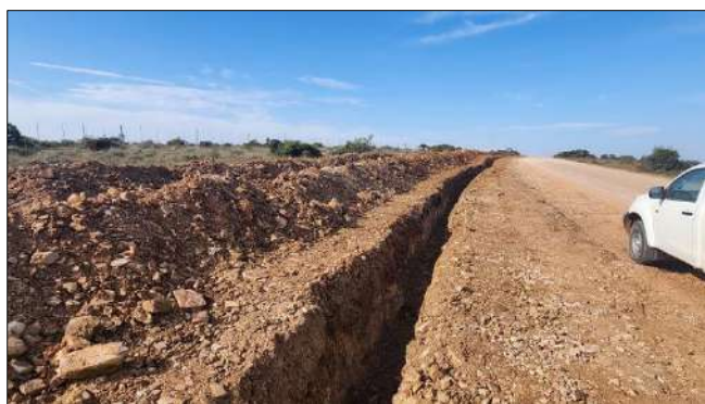
Photo 6a: MVA cable trench between substation and turbines.
