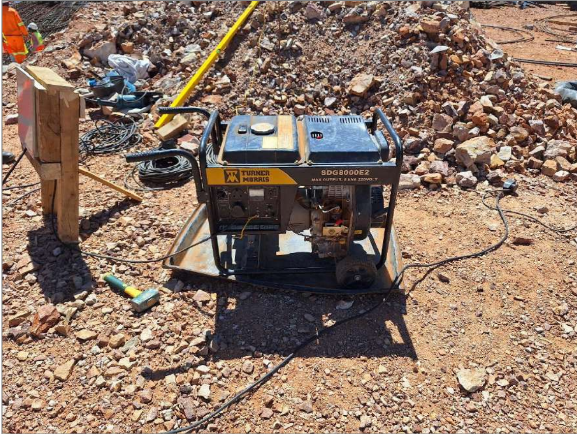
Figure 4: Use of drip trays under generators.
