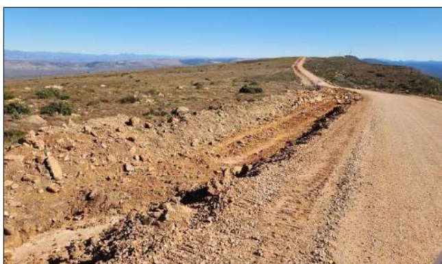
Photo 5a: Backfilled section of an MVA cable trench.
