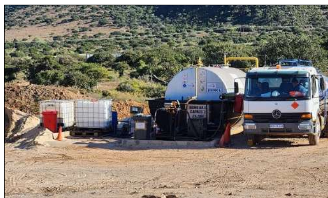
Photo 8a: Bunded fuel storage facility at the temporary laydown area.
