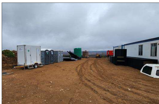
Photo 6c: Chemical ablutions available at the Vestas office / laydown area.
