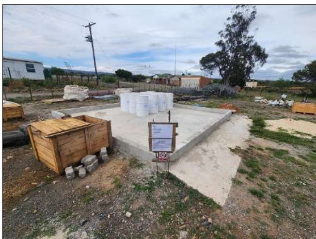
Photo 3c: Bunded platform for storage of transformer oil at Wolwefontein laydown area.
