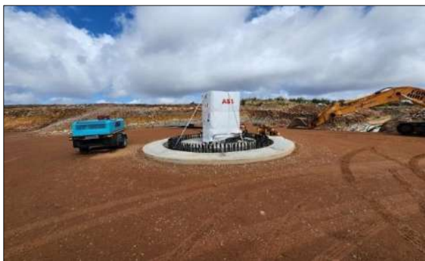
Photo 5a: Drip tray observed in use for mobile generator.
