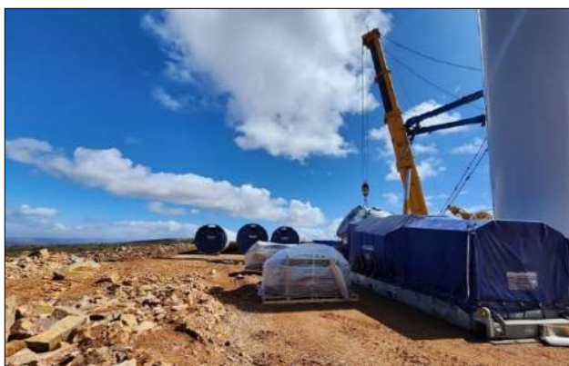
Photo 3a: Turbine components stored on site pre-assembly.
