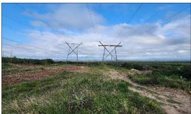
Photo 7d: View south towards Grassridge SS at the outage site where the CR line will tie in to the existing 132kV line.
