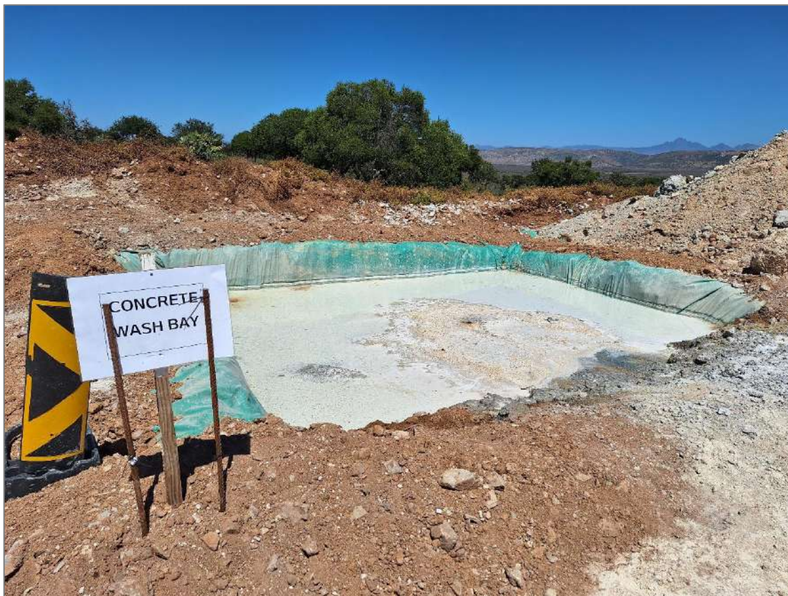
Figure 2: Dedicated concrete wash bay
