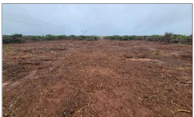
Photo 3d: Vegetation cleared unnecessarily at five tower footprints between CR112 and CR117.
