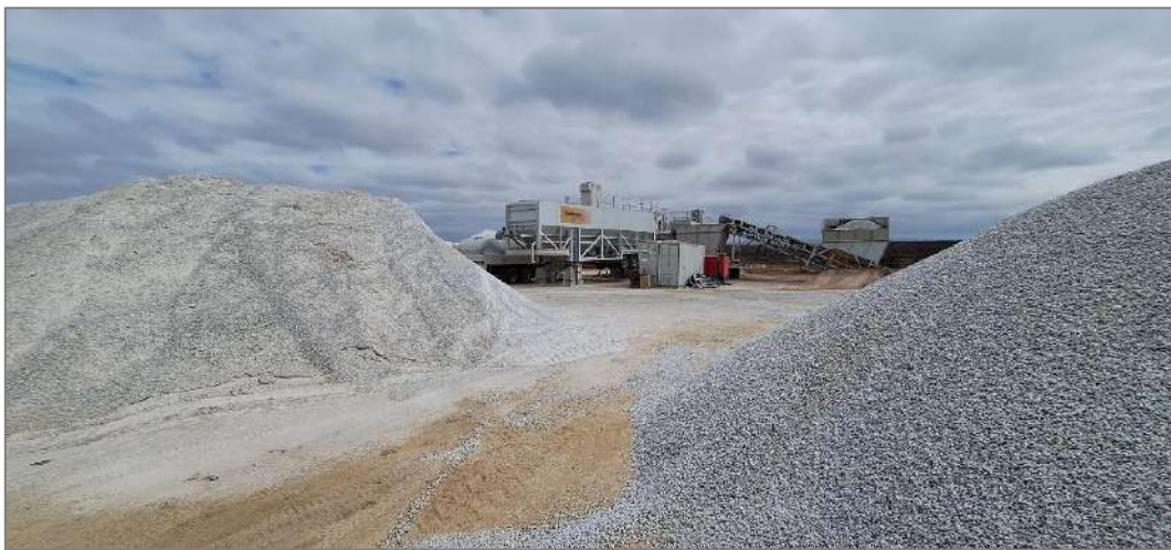
Figure 7: Operational batch plant.
