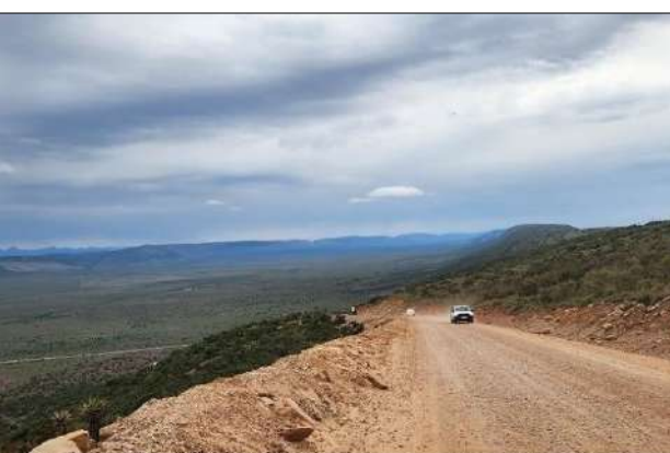
Photo 8b: State of gravel road section before the transition to the paved surface section which adjoins the R75 tar road.
