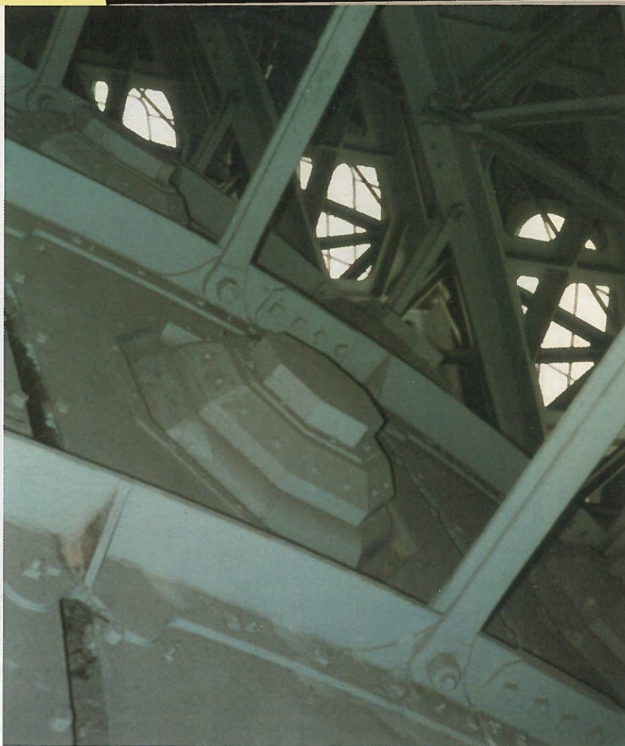
Cast iron modules, some as deep as 10 feet and weighing 10 tons, form the internal structure of the dome. Castings show remarkable dimensional tolerancing.
