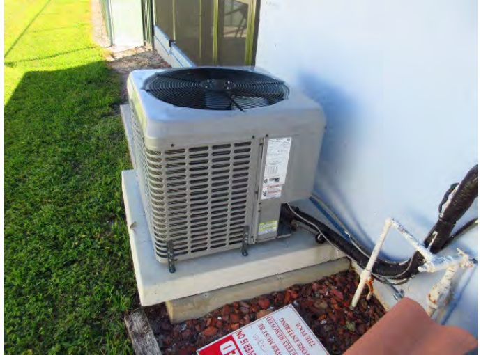
VIEW OF HVAC EQUIPMENT
