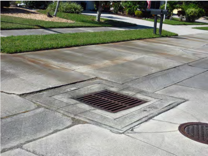
VIEW OF STORM WATER INLET
