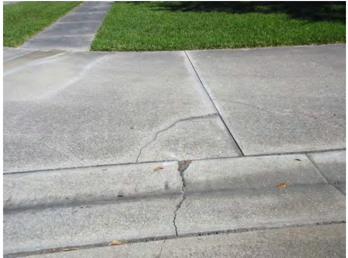
VIEW OF DAMAGED CONCRETE PAVEMENT
