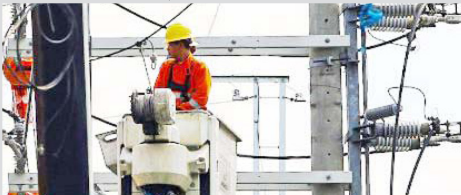
ENERGY NEEDS. An engineer of Manila Electric Company (Meralco) on a boom lift inspects electric posts along New York Street in Cubao, Quezon City in this May 30, 2024 photo. The bill renewing the Meralco's franchise for another 25 years has hurdled committee level at the House of Representatives. (PNA photo by Joan Bondoc)
