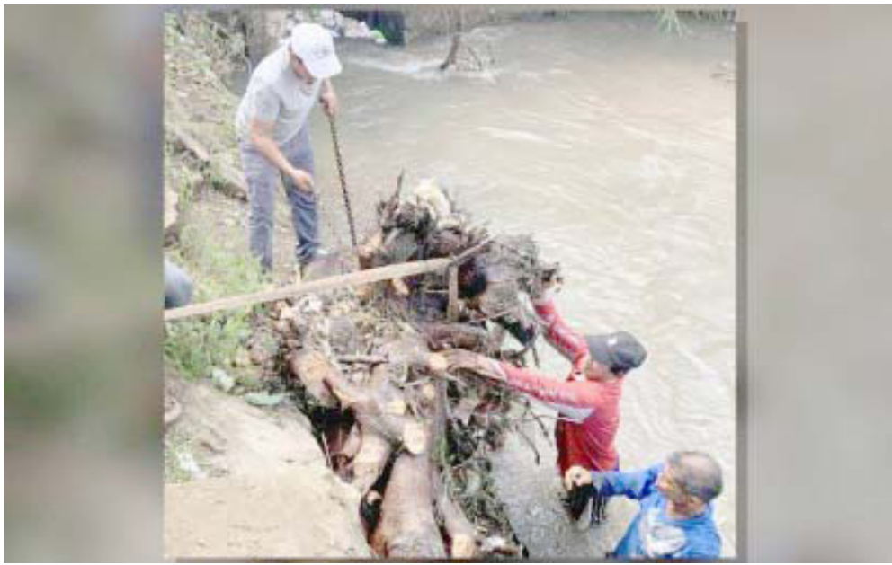
CLEAN-UP WORKS. National Irrigation Administration (NIA)-Calabarzon personnel and members of irrigators associations conducting desilting and clearing operations along irrigation canals to remove debris and restore water flow after Super Typhoon Carina in this undated photo. NIA placed the estimated damage caused by 'Carina' to its irrigation systems at PHP29.1 million and approximately PHP111.81 million in agricultural losses, especially on rice crops. (Photo courtesy of NIA-Calabarzon)
