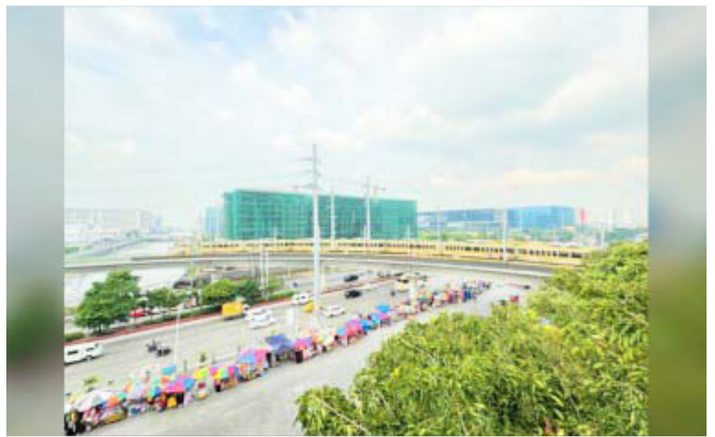
TEST RUN. The start of a series of test runs features a 2nd Generation train set that traversed the whole phase 1 of the LRT-1 Cavite Extension project on Tuesday (Dec. 19, 2023). The first test run aimed to provide a compatibility check and assess the interface between vital infrastructure components. (Photo courtesy of LRMC)
