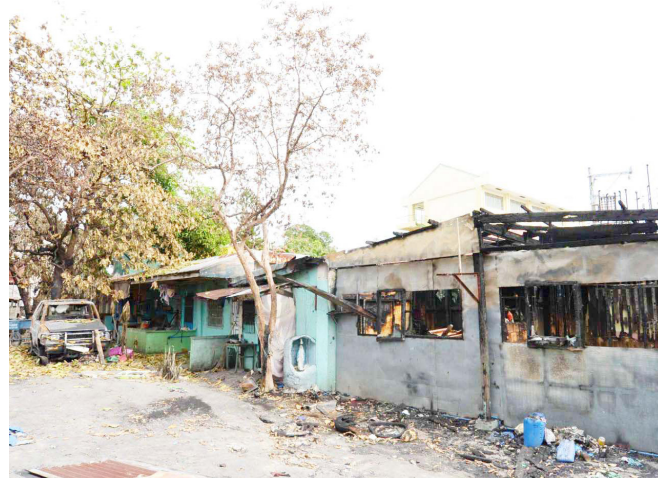
One of the structures that caught fire in Bacoor City. (OSBG Photo)
