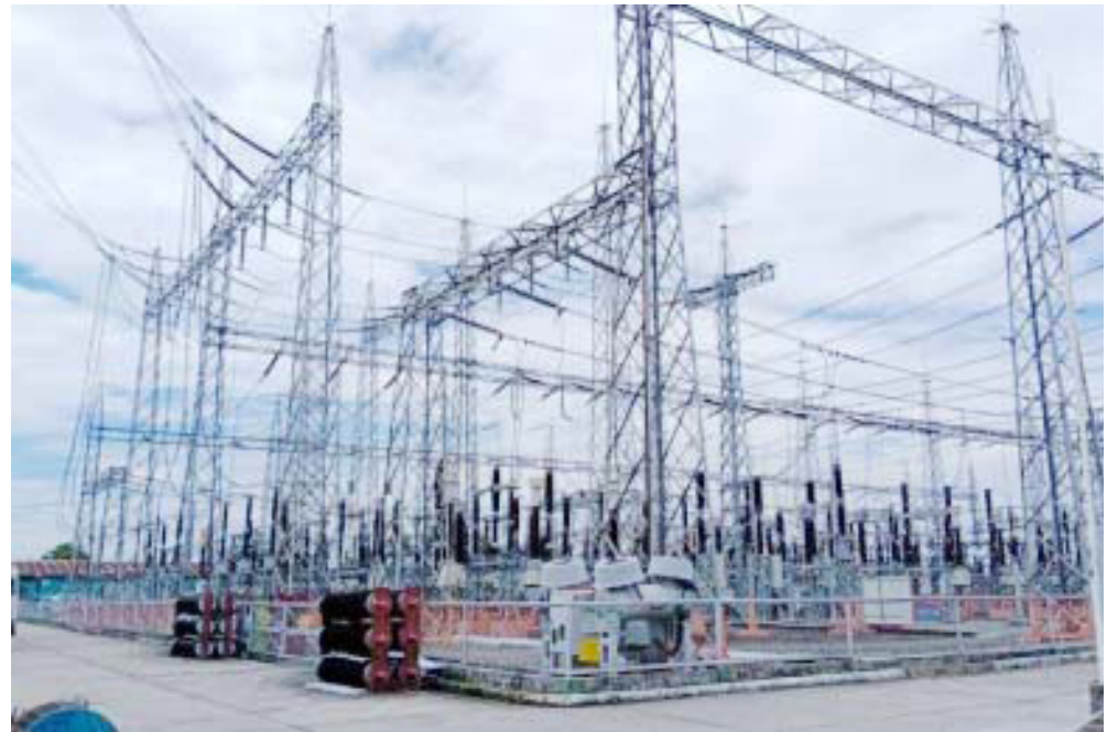
POWER UP. President Ferdinand R. Marcos Jr. inaugurated the new Mariveles-Hermosa-San Jose Transmission 500-kV project in Hermosa, Bataan on Friday (July 12, 2024). The Mariveles-Hermosa-San Jose Transmission Line will benefit about 59 million Filipinos in Luzon. (Malacañang Press Corps photo)
