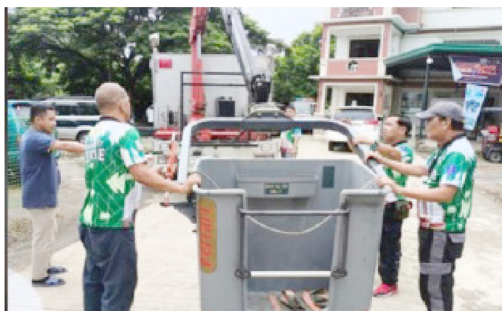
ADVANCED WATER MONITORING SYSTEMS. The automated rain gauge and water level monitoring system equipment developed by DOST-Advanced Science and Technology Institute (DOST-ASTI) and installed recently in two villages in Carmona City, Cavite province. Harley Margallo, spokesperson of DOST-Calabarzon's Public Affairs, Relations, and Communications Unit, said Wednesday (July 17, 2024) the technologies are expected to step up the disaster prevention and resilience efforts in the city. (Photo courtesy of DOST PARCU)
