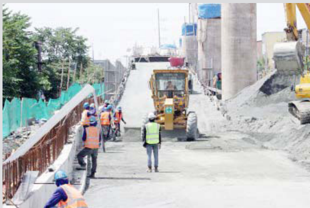
Construction site of the NLEX-SLEX Connector Project along Antipolo St. in Sampaloc, Manila (PNA file photo by Joey Razon)
