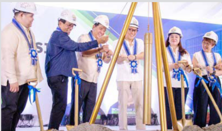
4PH PARTNERS. Department of Human Settlements and Urban Development Secretary Jose Rizalino Acuzar (2nd from left) joins Imus City Mayor Alex Advincula and Megawide Construction Corporation chief executive officer Edgar Saavedra at the groundbreaking ceremony for a housing project under the Pambansang Pabahay para sa Pilipino Program on Tuesday (May 28, 2024). Acuzar said the housing program has been rolled out and implemented in other areas. (Photo courtesy of the DHSUD)
