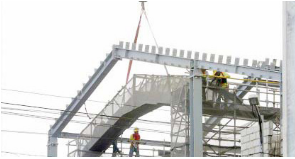
LRT-1 CAVITE EXTENSION PROJECT. Workers install a beam in the ongoing construction of the LRT-1 Cavite Extension project along Roxas Boulevard in Parañaque City on April 24, 2023. The closure of some portions of the road has been rescheduled due to adjustments in the construction timeline. (PNA photo by Avito Dalan)
