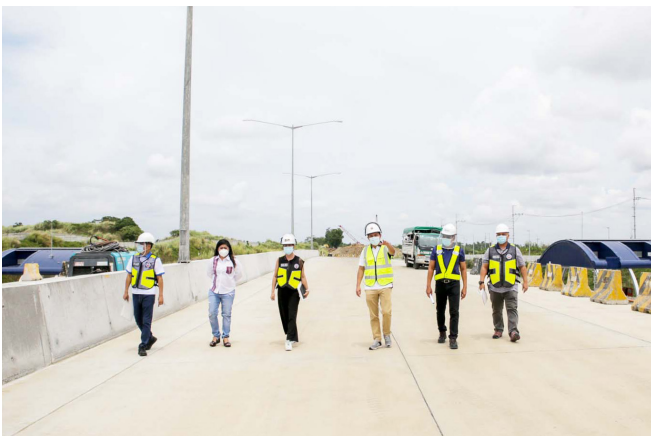
DPWH Sec. Mark Villar inspects CALAX Subsection 4. (from L-R) DPWH Director for PPP Service Alex Bote, BBB Chair Mae Lamentillo, DPWH Undersecretary for Planning and PPP Maria Catalina Cabral, DPWH Secretary Mark Villar, MPCALA Holdings Inc. Vice President for Tollways Development and Engineering Art Monge and DPWH OIC Chief, PPP Service, Engr. David Galang. (Photo & caption: MPTSouth)
