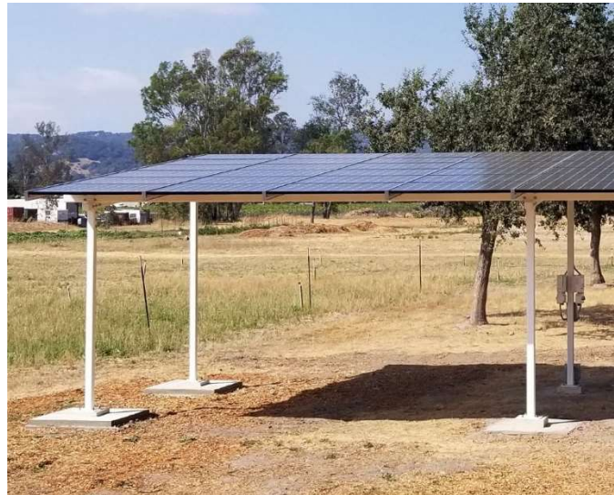
Figure 1 Photo provided courtesy of Solar Carports Direct
