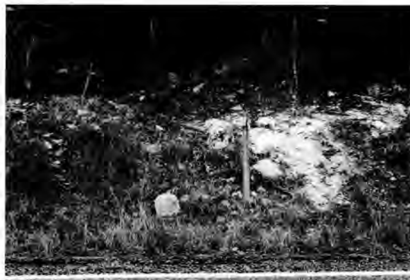
Figure 5. White fill material in looters' hole on highway Right-of-way. Note large rock near reflector that could roll onto highway.
