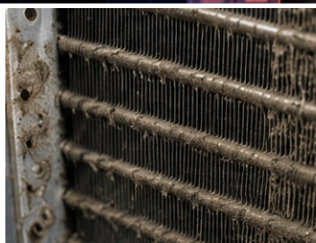
DIRTY COILS TRAP HEAT
