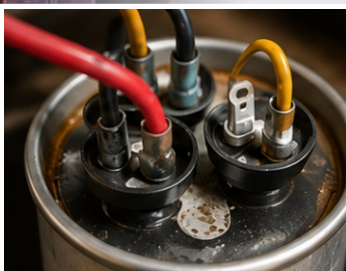
WEAK COMPONENTS OVERHEAT
