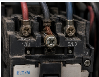
LOOSE CONNECTIONS CREATE MORE HEAT
