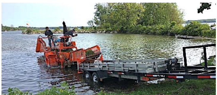
With the drum gone, the trailer can back down to the water's edge.
