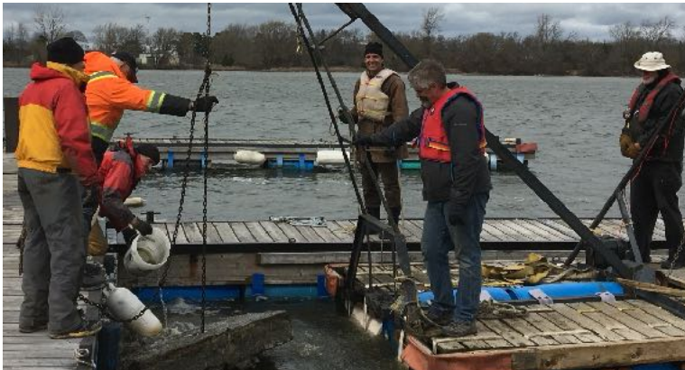
After last spring's ice movement, some D-dock anchors required re-positioning to bring the dock back into alignment. Above, the team removes mud from an anchor.
