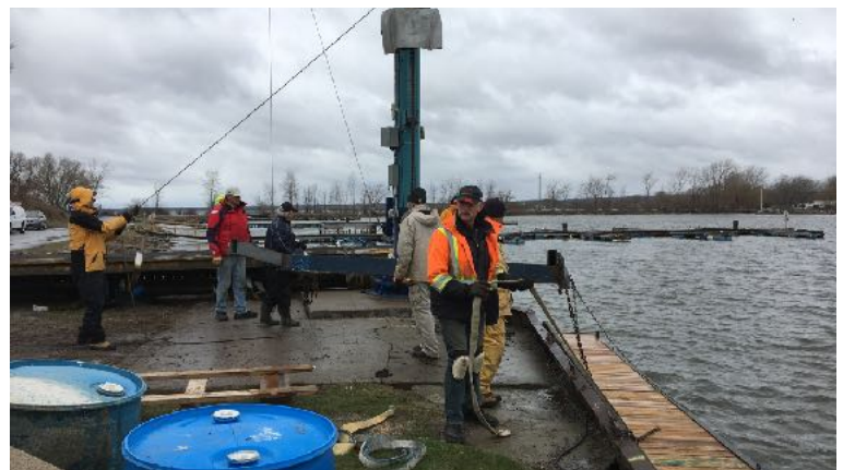
After last year's massive dock construction effort, only one new finger section was required this spring.
