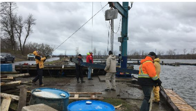
Launching the new finger dock at the mast crane. This section was constructed during the previous work party.
