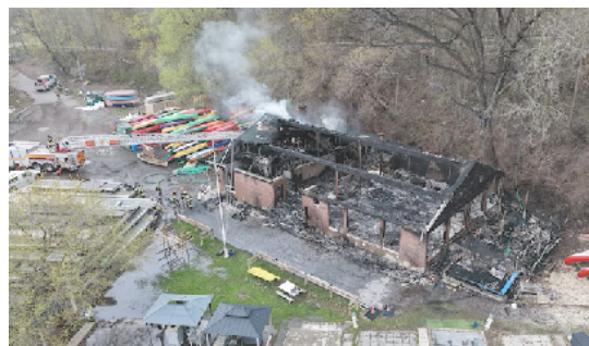
Remains of the building following the fire.
