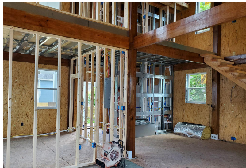
The recently updated Louisiana statewide building code is now one of the most stringent codes in the country
