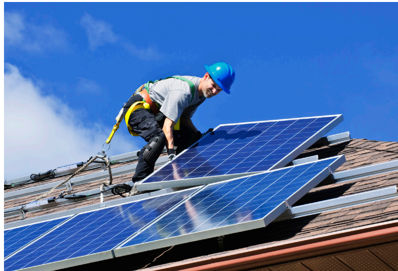
The Solar for All program presents a unique opportunity to combine rooftop solar installations with roof upgrades
