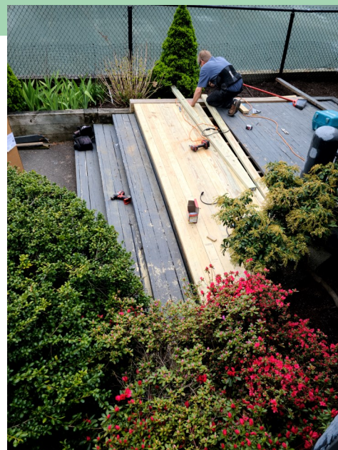
You will be seeing repairs happening around the property as we work towards the opening of the summer season.
