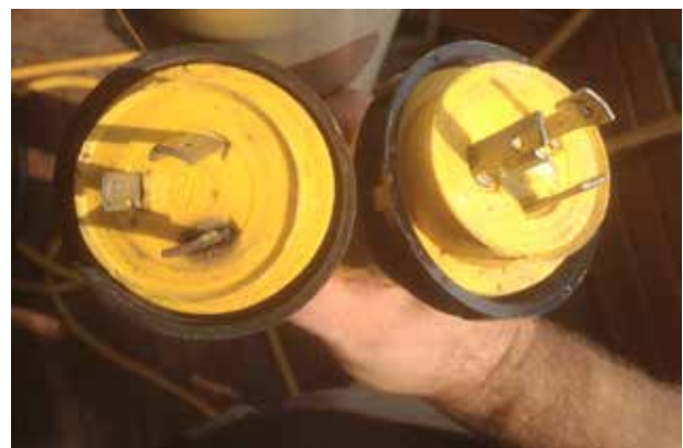
Cord end on the left is heat damaged
