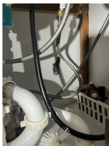
6.3 Item 1 (Picture) under kitchen sink on back wall
