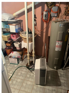
5.2 Item 1 (Picture) Water heater missing TPR valve
