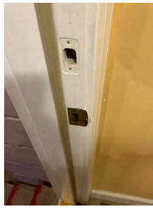
2.1 Item 2 (Picture) garage/laundry room door
