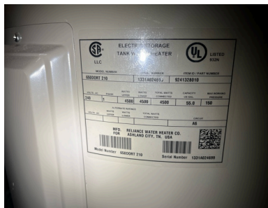
5.2 Item 2 (Picture) water heater nameplate
