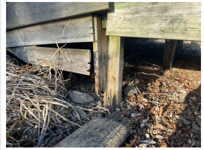
2.3 Item 6 (Picture) lake dock post deterioration
