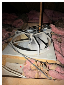
7.5 Item 1 (Picture) Attic whole house fan
