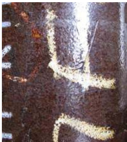
API 5L Piping
