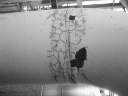
FIGURE 1: Poor field joint repair
