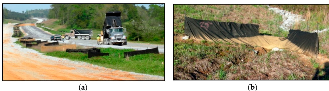
Figure 7. (a) In-field installation of silt fence ditch checks with weirs, (b) single silt fence ditch check with weir installed in field.
