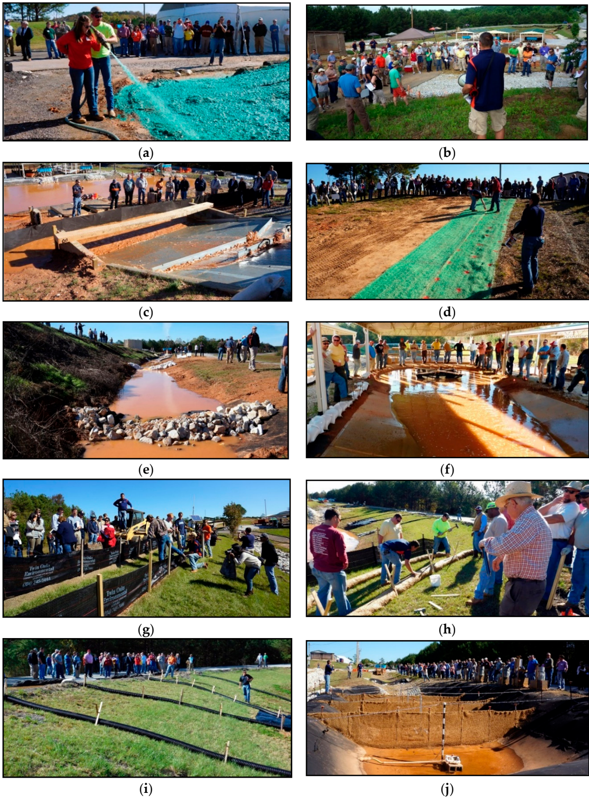
Figure 2. Demonstration stations at the AU-ESCTF: (a) Station A: Hydroseeding, (b) Station B: Construction Exit Pad, (c) Station D: Sediment Barriers, (d) Station E: Erosion Control Blankets, (e) Station F: Ditch Check Practices, (f) Station G: Channelized Flow Demonstration, (g) Station J: Silt Fence Installation, (h) Station K: Slope Interrupters, (i) Station L: Slope Drains, (j) Station M: Sediment Basin.
