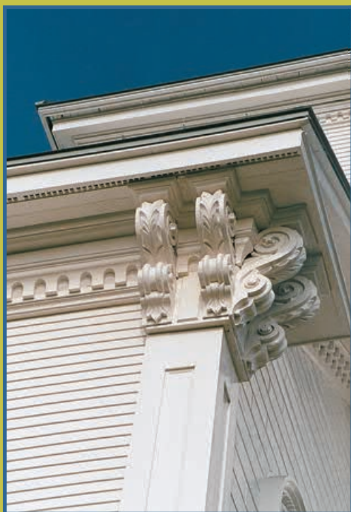
Photo above shows the use of Spectis custom bracket and pilaster.
