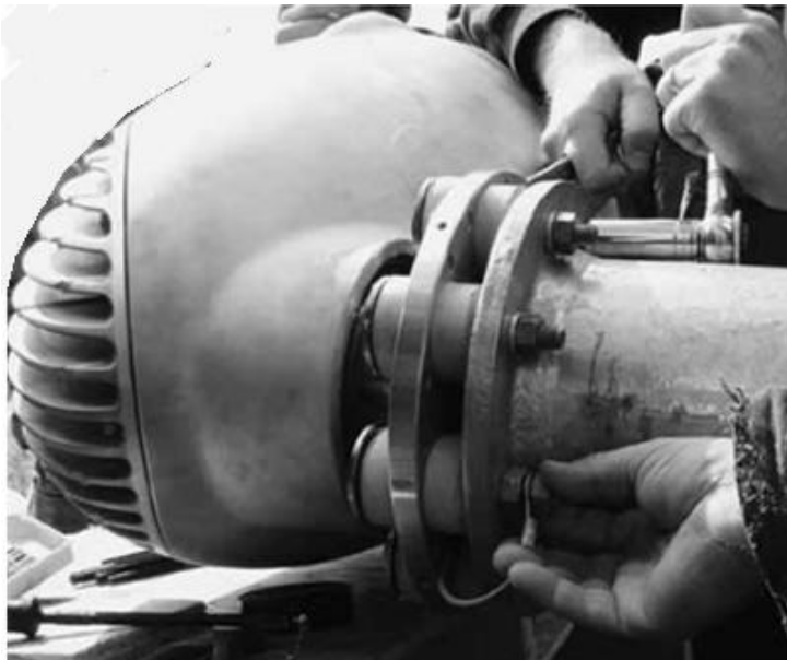
Figure 9 Grounding turbine to tower
