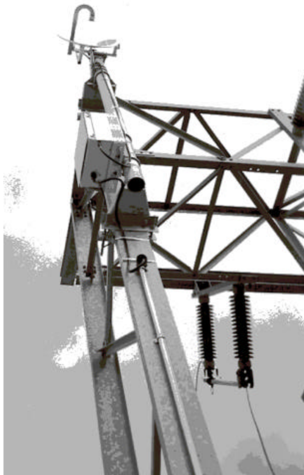
Figure 17-5: 6 GHz Microwave Terminal Mounted on Substation Box Structure
