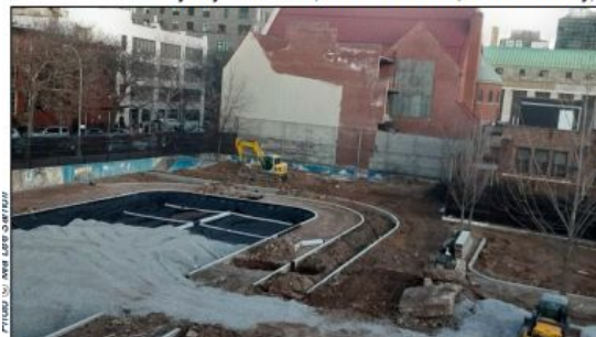
Construction workers used bulldozers to spread gravel at P.S. 38's new playground.
