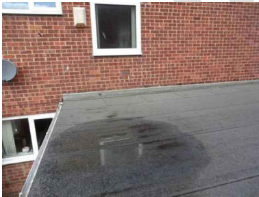
VIEW FULL SIZE Ponding was seen
