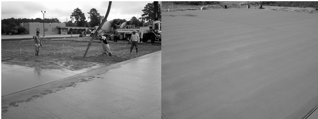
Fig. 2. Pouring concrete for the truck stop (left) and concrete surface of the truck stop after setting (right).
