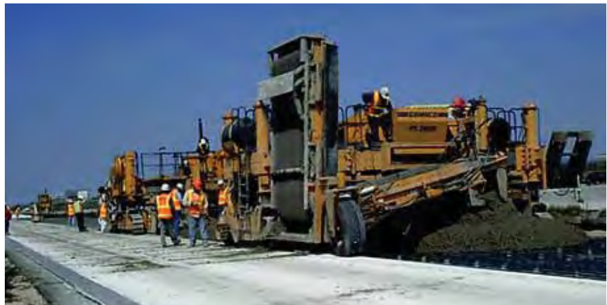
The laying of pavement on the IH-10, Texas, USA, using EMC Technology
