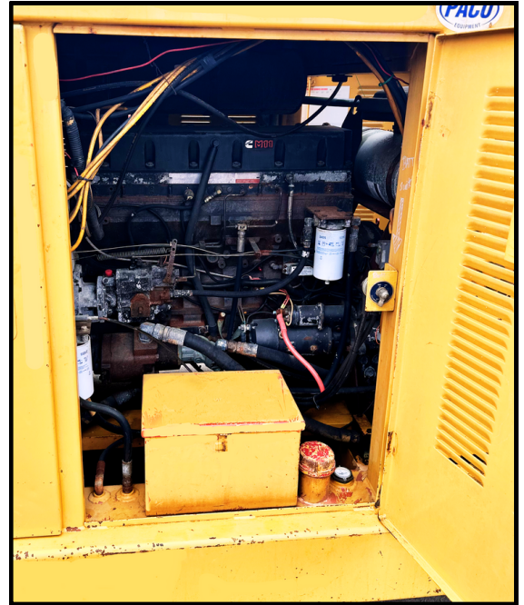
Photo 2 of 3 - Power Unit Cummins Engine
