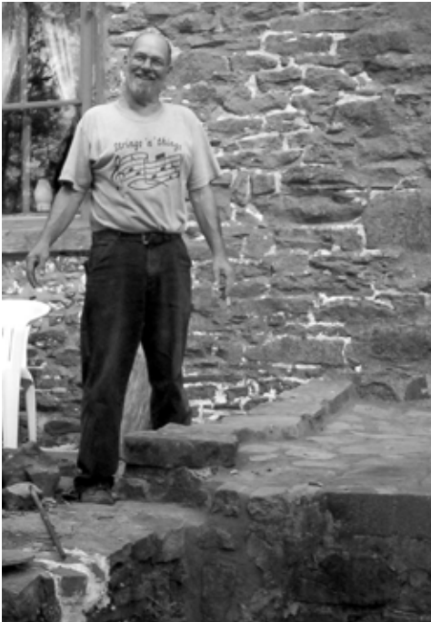
Gordon Allem repaired the stone work on the end of the porch
