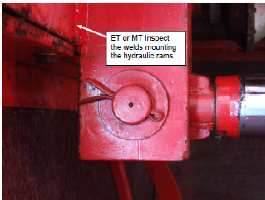
Fig 11: Welded brackets holding the central tower elevation rams.
