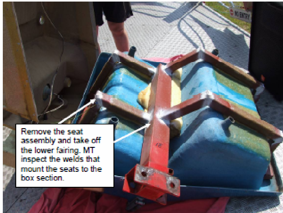
Fig 12: View of a chair assembly with lower fairing removed to gain access to the structure.
