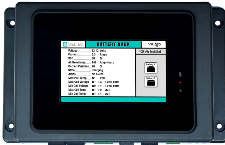
Figure 1. Touchscreen Showing Battery Bank page
