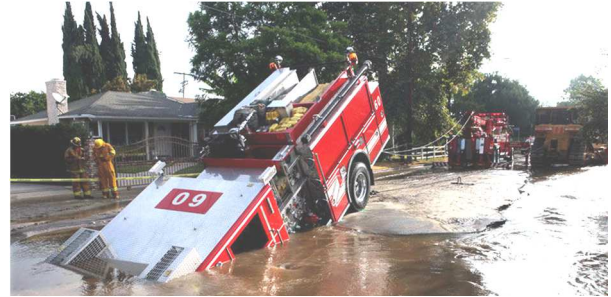
A $500,000 fire truck damaged in a sinkhole created by a corroded water main.
