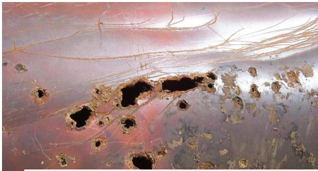
A close-up of an underground storage tank. Corrosion has compromised its integrity. How much are the associated cleanup costs??
